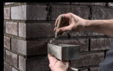
The vertical joints can be finished more easily with a smaller pointing trowel.
