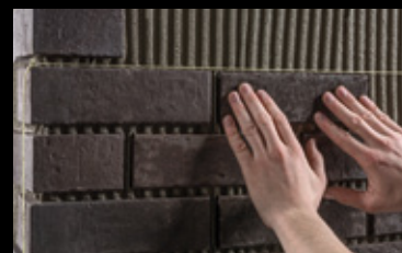
Use a string to plumb the clinker area. The clinker slips are pressed into the adhesive bed.
